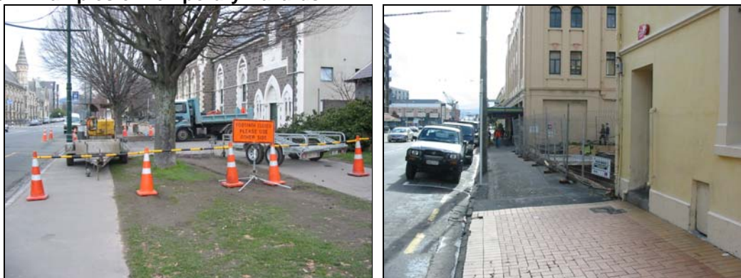
Figure PL16.1 Examples of Temporary Hazards
